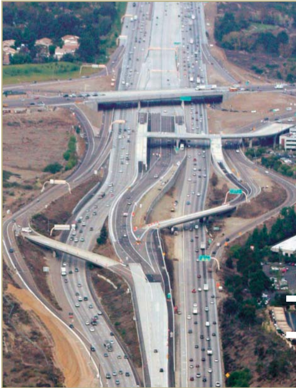
Construction of the DAR at the Sabre Springs/Peñasquitos Transit Station: aerial view looking north.
