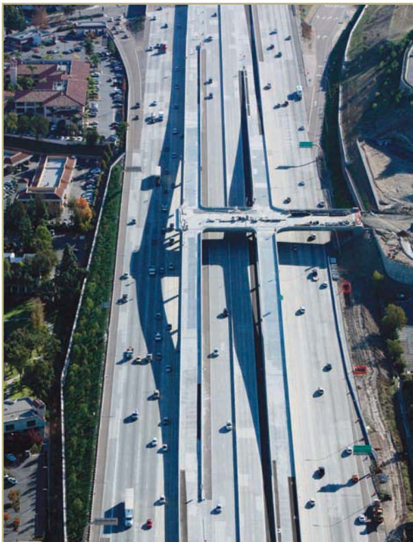
Construction of the DAR at the Rancho Bernardo Transit Station: aerial view looking south.
