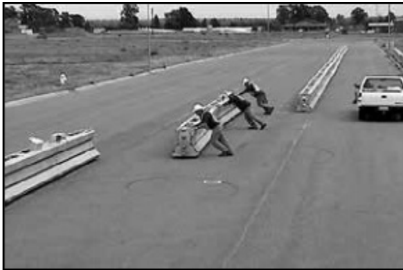
Figure 5. Relocate the section, or in this case Multi-section (56') to the desired position. Typically two people can easily control and move a single link section (28') and 3 people are typically used to move a multi-section (56') as shown above.
