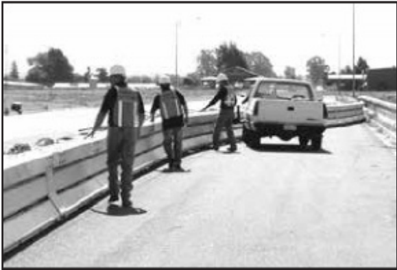
Figure 15: As the wall is being repositioned personnel lower each section at its final deployment or storage position.
